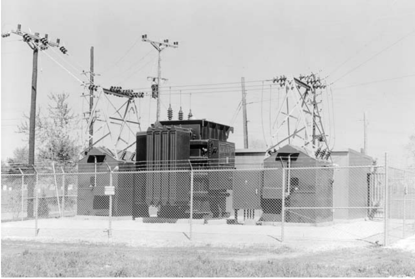
FIGURE 2.27 A distribution substation operating 34.5/4.16-kV voltage level. (Union Electric Company.)
