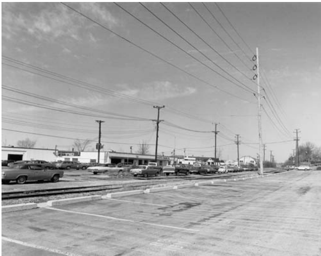
FIGURE 2.22 A typical 34.5-kV line with a double circuit and wood poles. It also has a 4.16-kV underbuild line and a 34.5-kV switch. (Union Electric Company.)
