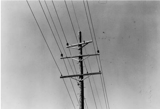
FIGURE 2.21 A 34.5-kV line with a single circuit and wood poles. It also has a 12.47-kV underbuild line and 34.5-kV switch. It has an old style construction. (Union Electric Company.)
