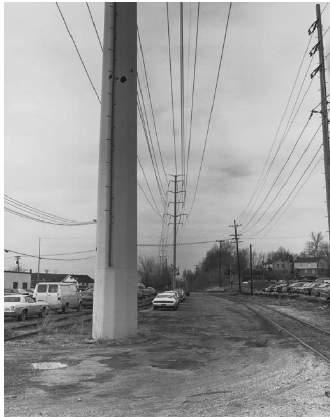
FIGURE 2.6 A double circuit 138-kV line built by using steel poles, having two 138-kV circuits underbuild. (Union Electric Company.)
