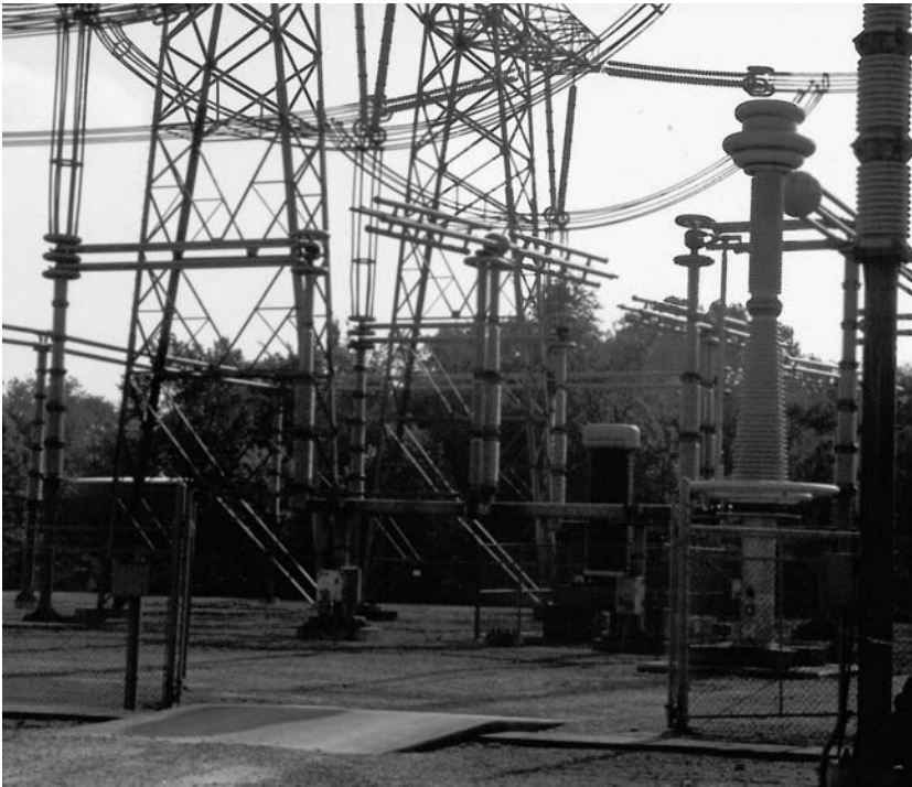
FIGURE 6.11 A 800-kV disconnect switch on the ac side at the same converter station.
