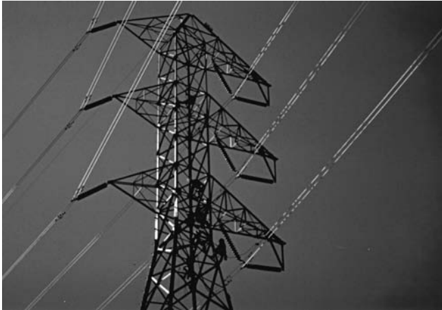
FIGURE 2.14 A typical 230-kV transmission line steel tower with bundled conductors and double circuit.
