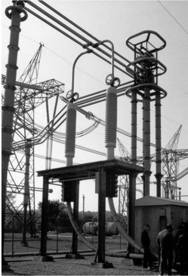
FIGURE 6.12 800-kV risers on the ac side at the same converter station.
