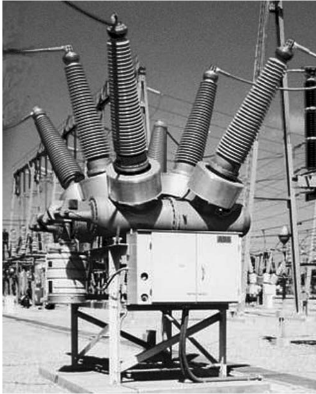
FIGURE 10.2 Three-pole-operated 245 kV SF 6 dead-tank circuit breaker fitted with 80-kA interrupters. (Courtesy of ABB Corporation.)
