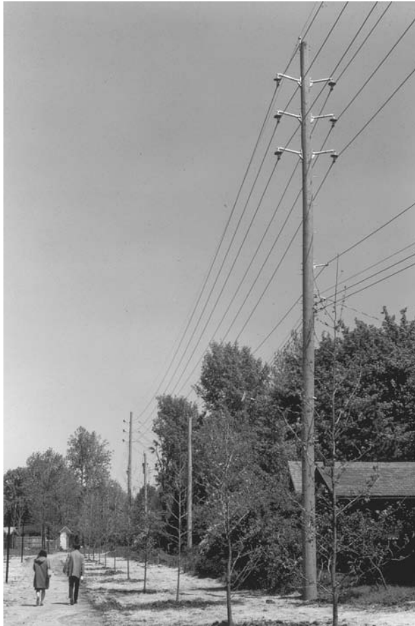
FIGURE 2.20 A typical 34.5-kV line with a double circuit and wood poles. It has a newer style construction. (Union Electric Company.)
