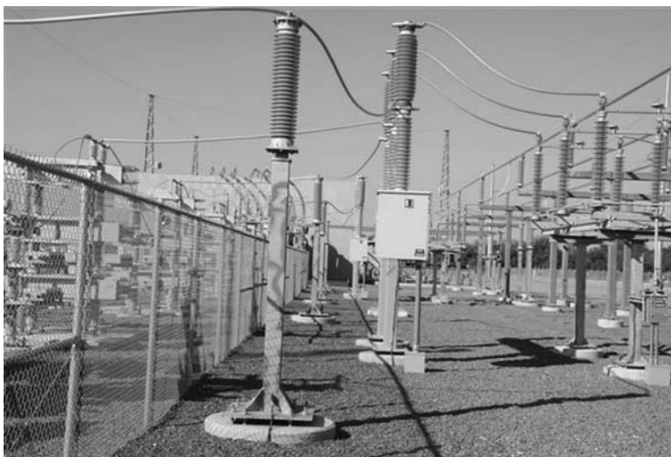
FIGURE 10.3 Single-pole-operated 138 kV SF 6 live-tank circuit breakers. (Courtesy of ABB Corporation.)
