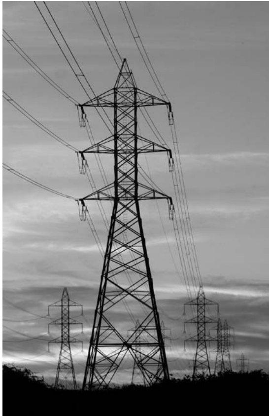
FIGURE 1.2 A three-phase double-circuit transmission line made of steel towers.
