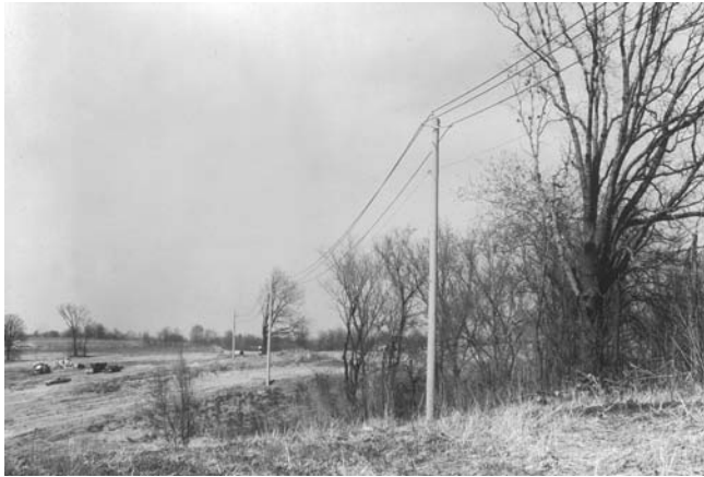
FIGURE 2.23 A typical 12.47-kV line with a single circuit and wood pole. It has a newer type pole top construction. (Union Electric Company.)
