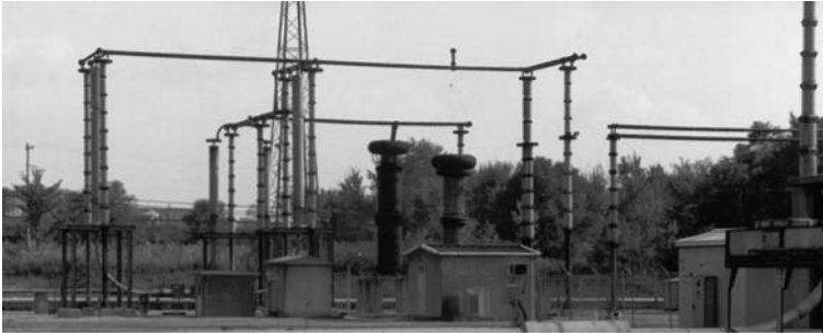
FIGURE 6.10 800-kV dc terminals of a converter station.
